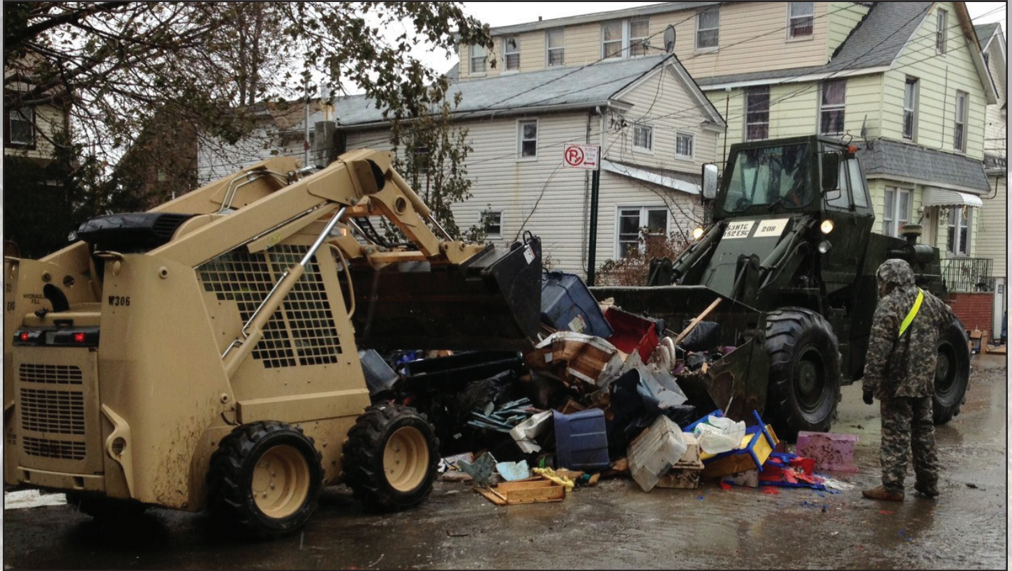
Members of the New York Army National Guard's 204th Engineer Battalion work to clear streets in Far Rockaway on Nov. 7. The Queens community was battered by Hurricane Sandy when it hit on Oct. 30. The Guard engineer Soldiers have been working to clear debris left by the storm. Photo courtesy of 204th Engineer Battalion.
