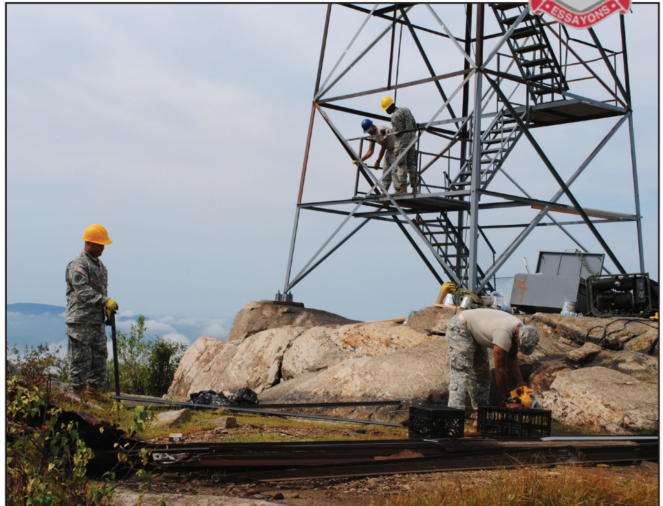
Staff Sgt. Marco Padilla and Spc. Osse Jean-Pierre of the 1156th Engineer Company, New York Army National Guard, repair and replace railings on the Mount Beacon fire tower Sept. 7, 2012 (Photo by Army Sgt. 1st Class Thomas Wheeler, 138th PAD)
