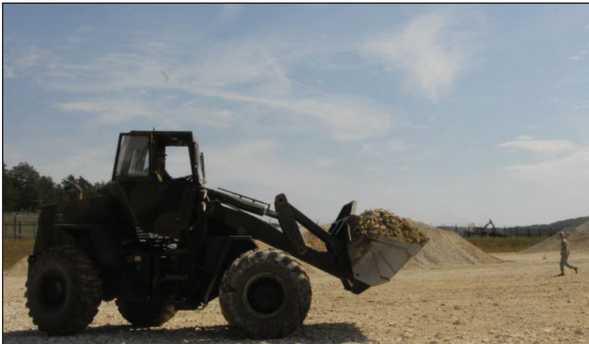
HOHENFELS, GERMANY-- A construction vehicle transports gravel to the helicopter landing zone at the Joint Multinational Readiness Center here, Aug. 15. Seventy-eight New York Army National Guard Soldiers with the 827th and 152nd Engineer Companies from the 204th Engineer Battalion, Walton, N.Y. traveled to Hohenfels to aid in troop construction projects on the base's pre-deployment training area as part of their annual training, August 5-24.
