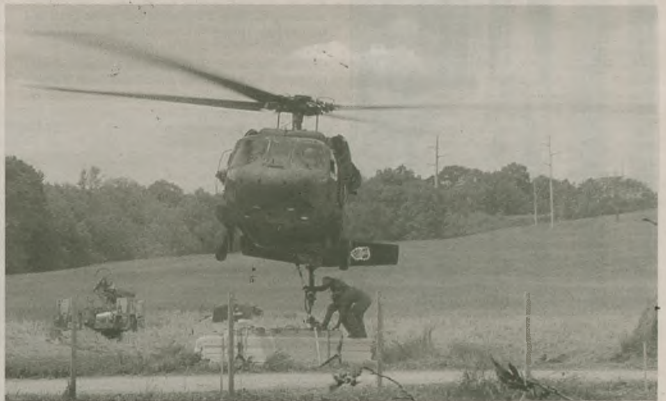
Crews from the Albany area's 3 rd Battalion, 142 nd Assault Helicopter Battalion prepare to hookup drilling and support equipment for the Department of Transportation's engineering assessment of the Delmar landslide over the Memorial Day Weekend. The slingload operation was the only practical method of delivering the drilling equipment to the landslide site to assess the soil's stability. The National Guard members were called to State Active Duty for the holiday weekend for the mission to support the state's emergency management office. Photos by Lt. Col. Paul Fanning.
