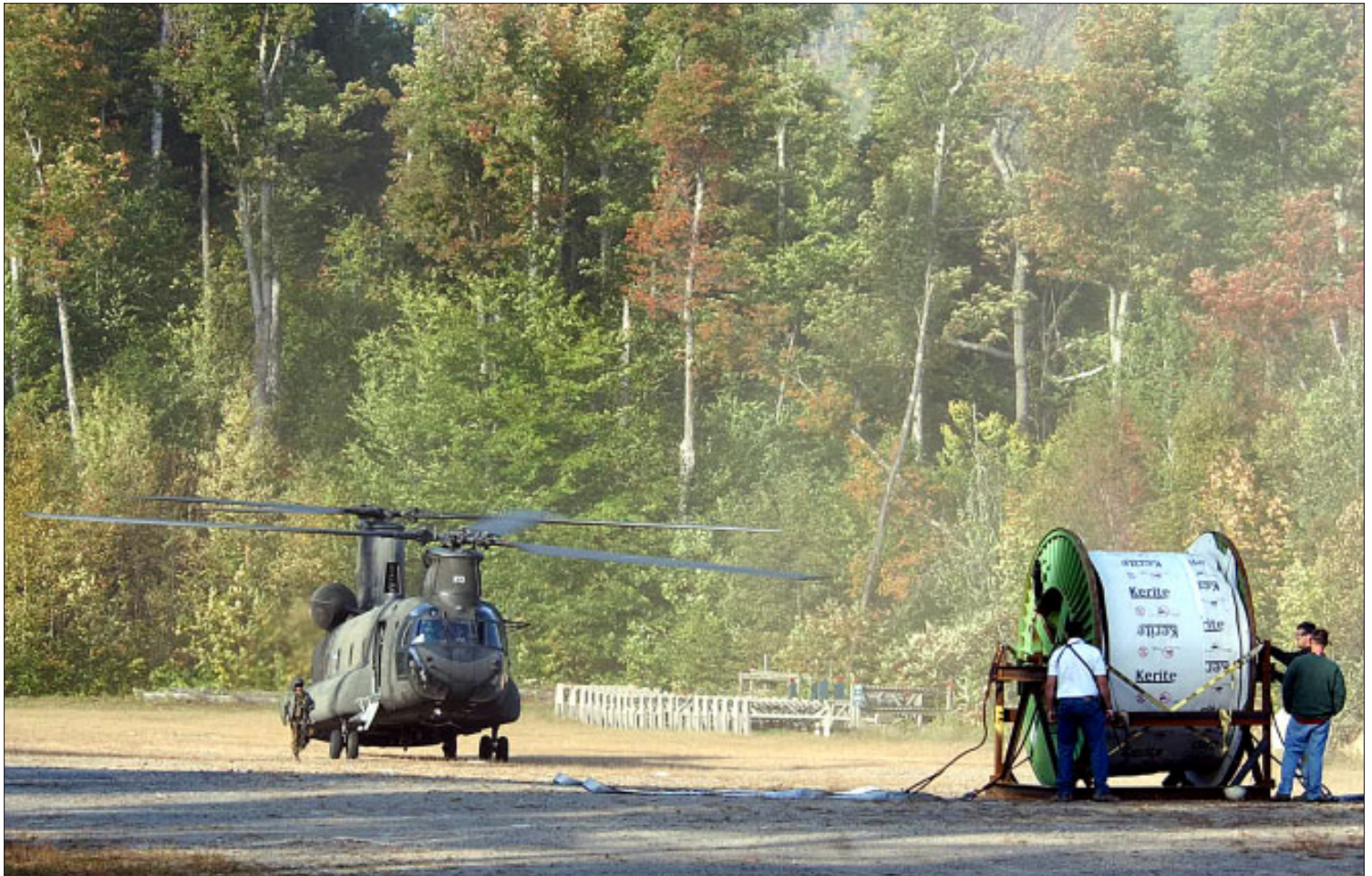
A CH-47 Chinook from Army Aviation Support Facility 2 in Rochester lands at Whiteface Mountain Sep. 29 to lift a 19,000 pound spool of power cable to the mountain's summit. The mission was organized through the NY National Guard's GUARDHelp program; read the full story on page six (Photo by Staff Sgt. Mike R. Smith, Guard Times Staff)
