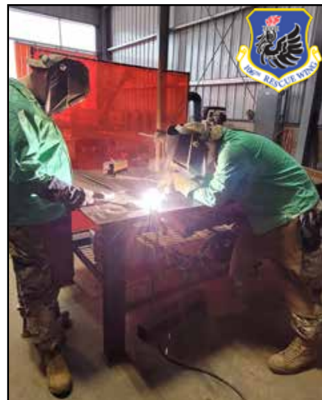
106th Rescue Wing structural specialist engineers practice welding at the Silver Flag exercise at Tyndall Air Force Base, Panama City, Florida, Jan. 10, 2022. Courtesy photo.
