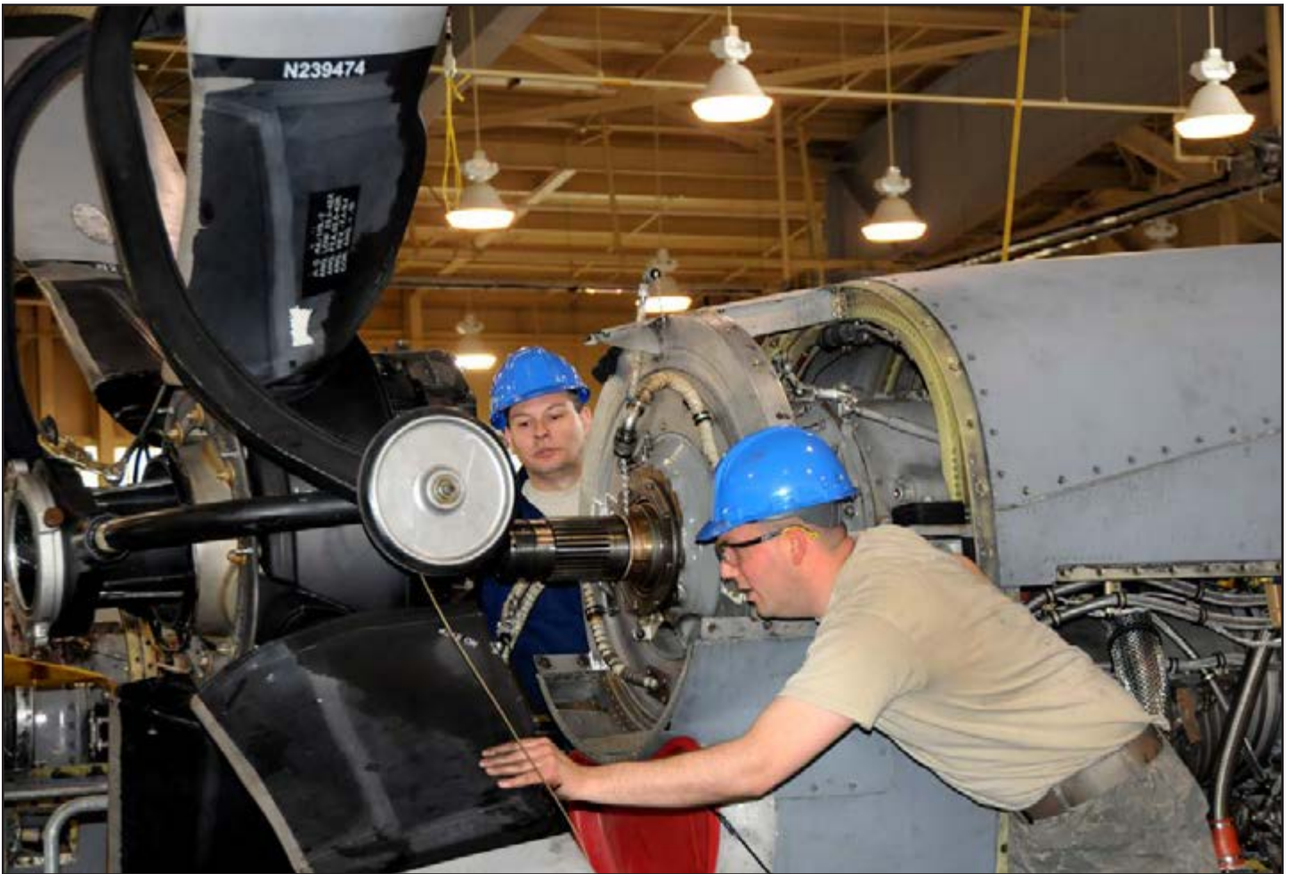
New York Air National Guard Tech. Sgt. Aaron Clause, right, and Tech. Sgt. Dan Weiser guide a prop onto a newly installed C-130 T56 engine. The Air National Guard's 107th Airlift Wing's maintenance team installed the rebuilt engine during scheduled maintenance May 4 to prepare the wing aircraft for deployment to Afghanistan.
