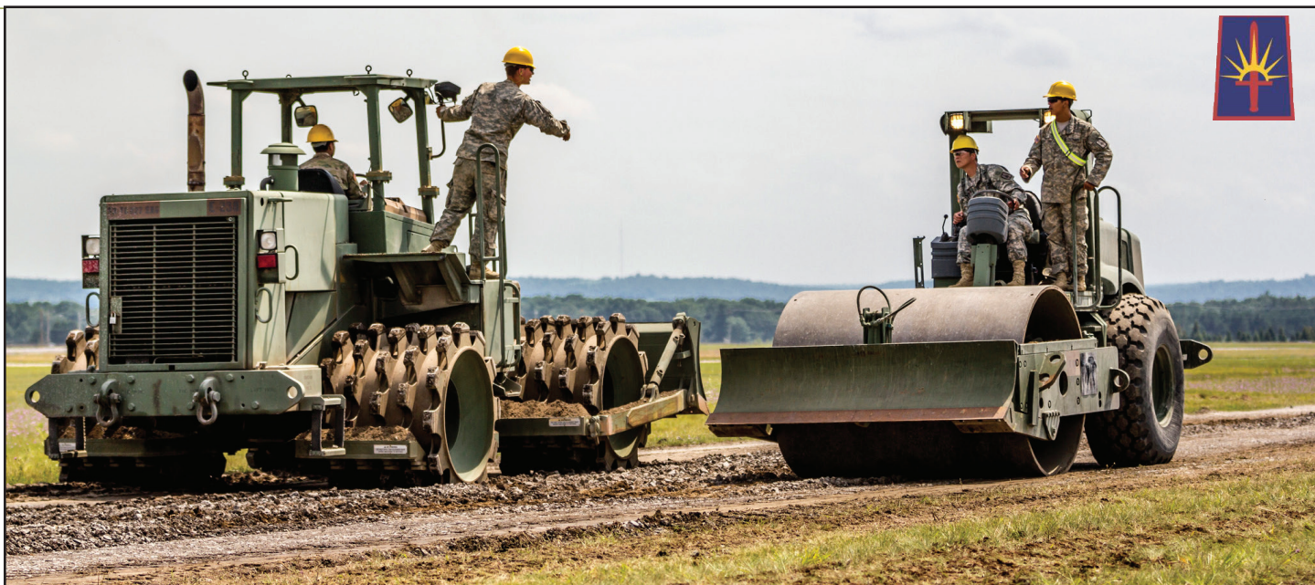
Soldiers with the 827th Engineer Company, 204th Engineer Battalion, tear apart and regrade a road at Fort Drum, N.Y., July 19th, 2017. Photo by Sgt. Harley Jelis. Opposite page: 1156th Engineers attach a piece of siding to a shed. The Soldiers were part of four construction projects during annual training that honed skills while completing projects for the post. Photo by Spc. Amouris Coss, 138th Public Affairs Detachment.
