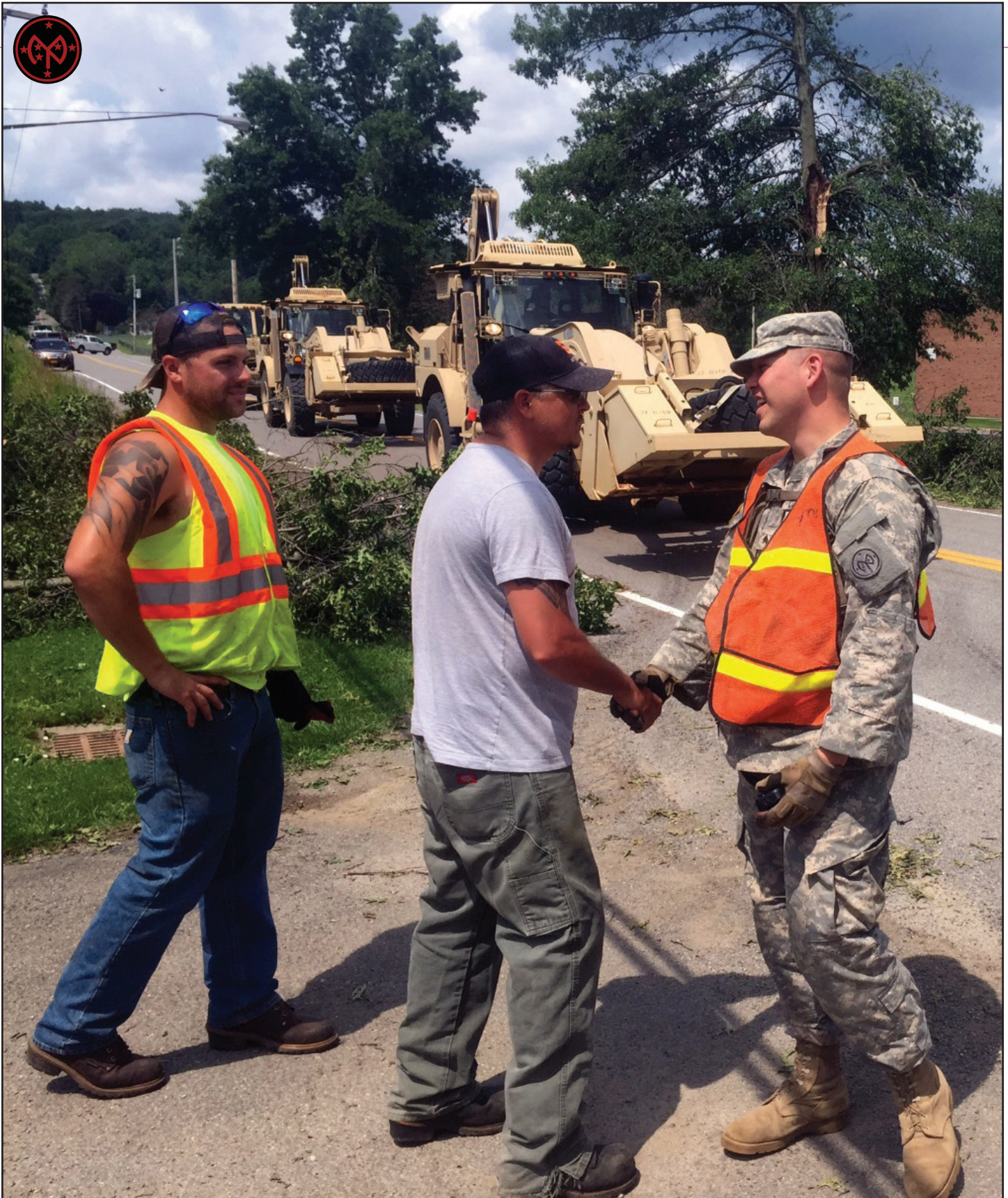
Sgt. Raymond Faltisco conducts initial linkup with Erie County Highway Department counterparts near Holland, New York following tornado storm damage on July 20, 2017. Faltisco, from Buffalo, New York, joined other New York Army National Guard Engineers assigned to Company A, 27th Brigade Special Troops Battalion as part of a 100-member joint National Guard response element to assist local emergency responders with recovery efforts. A tornado touched down in Erie County in Western New York State July 20, leaving an initial 20,000 residents without power and downing power lines and trees, blocking local roads with debris. Photo courtesy of New York Army National Guard Maj. Justin Courts.
