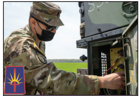
Staff Sgt. Christian Cuesta, a multichannel transmission systems operator-maintainer and the team leader at Regional Support Center Panther, assigned to Bravo Company of the 101st Expeditionary Signal Battalion, prepares a generator in North Vernon, Ind., April 20, 2021.
