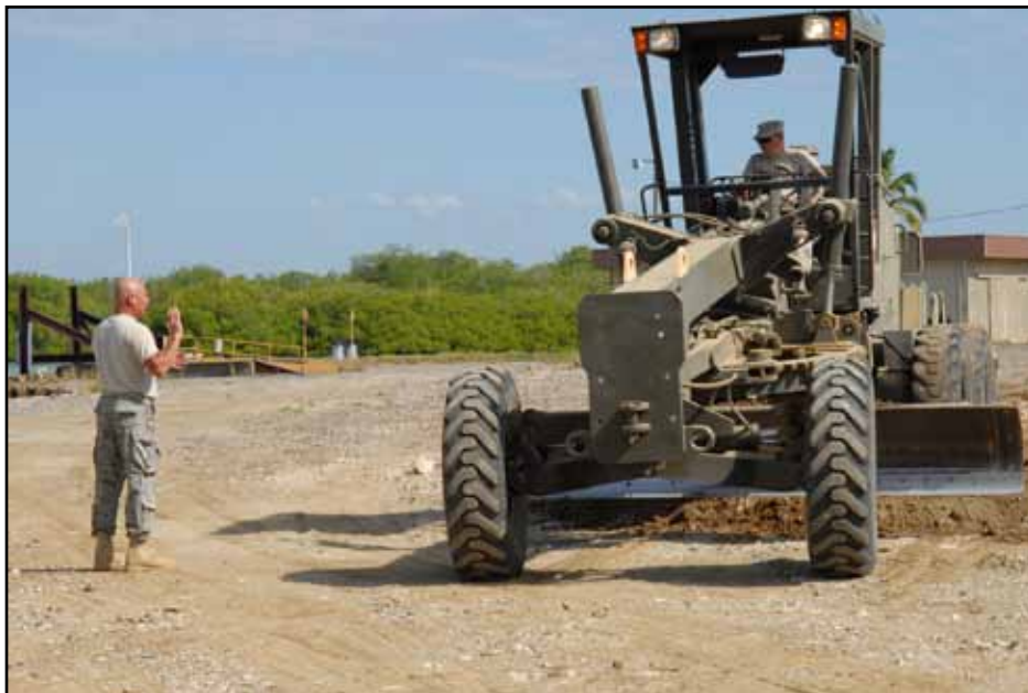
Air Force Master Sgt. James Vella directs Air Force Tech. Sgt. John Gentile while leveling a piece of land during a road improvement project near the U.S. Naval Station Guantanamo Bay airfield, Jan. 26, 2010. Vella and Gentile are with the 106th Civil Engineering Squadron of the New York Air National Guard.
