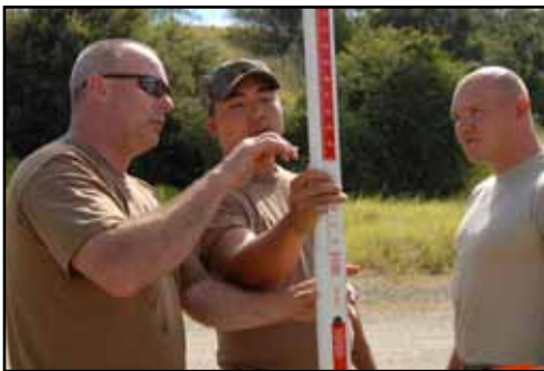
Air Force Master Sgt. Joe Casey (left) explains to Air Force Staff Sgt. Alex Chi and Airman 1st Class Sergey Klebleyev the process for surveying while completing a road improvement project near the U.S. Naval Station Guantanamo Bay airfield, Jan. 26. The Airmen are with the 106th Civil Engineering Squadron of the New York Air National Guard. The 106th is conducting a two-week deployment for training at Guantanamo Bay to assist in ongoing relief efforts for Operation Unified Response.
