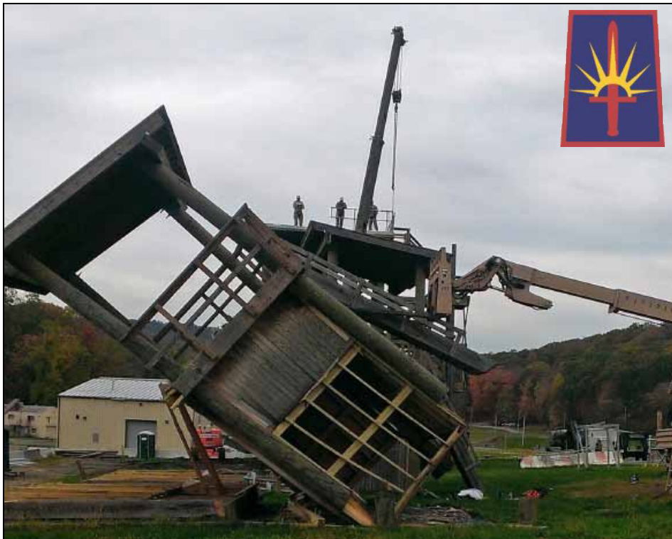
Making way for the construction of a new maintenance facility, New York Army National Guard engineers dismantle one of three rappel towers at the Camp Smith Training Site in late October 2014. The mission was one of several troop-labor projects that the Soldiers accomplished in the first week of their two-week annual training period. The Soldiers, who belong to the 1156th Engineer Company and the 204th Engineer Battalion, also installed better drainage, constructed sidewalks and dismantled an aging set of grandstands, along with other tasks.
